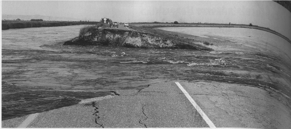
Figure 21 Regional Flooding In 2004, flooding on the Middle River near Holt, California, washed out this highway and covered a wide area with rushing floodwaters.
